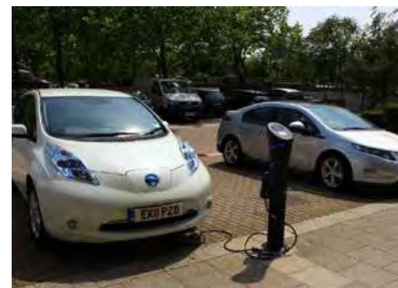
Electric car charging points
